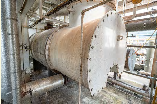
Waste Heat Boiler and Superheater
